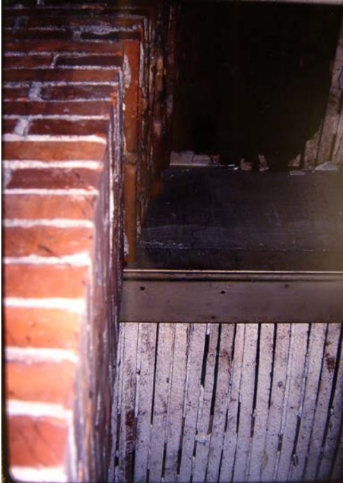
This photo from Bruce Banks shows a crooked chimney in the building. He said that was a result of its move across Rocky River.
