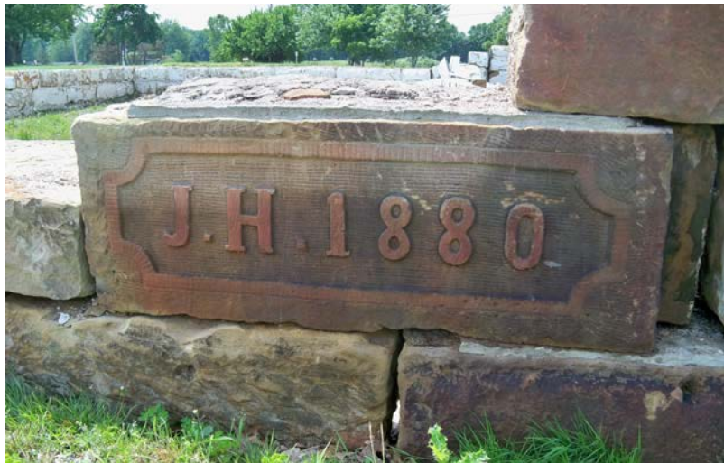
The stone with John Hall’s initials and the year of construction now sits on the northern side of what is left of the barn’s foundation rather than the western side, where Hall put it.
