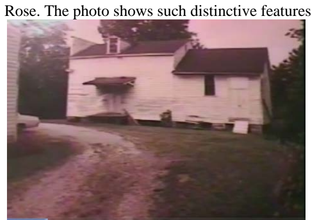
Another photo of the Granary from a Grand Pacific Junction video shows its deteriorated condition prior to renovation. Photo courtesy of Clint Williams
