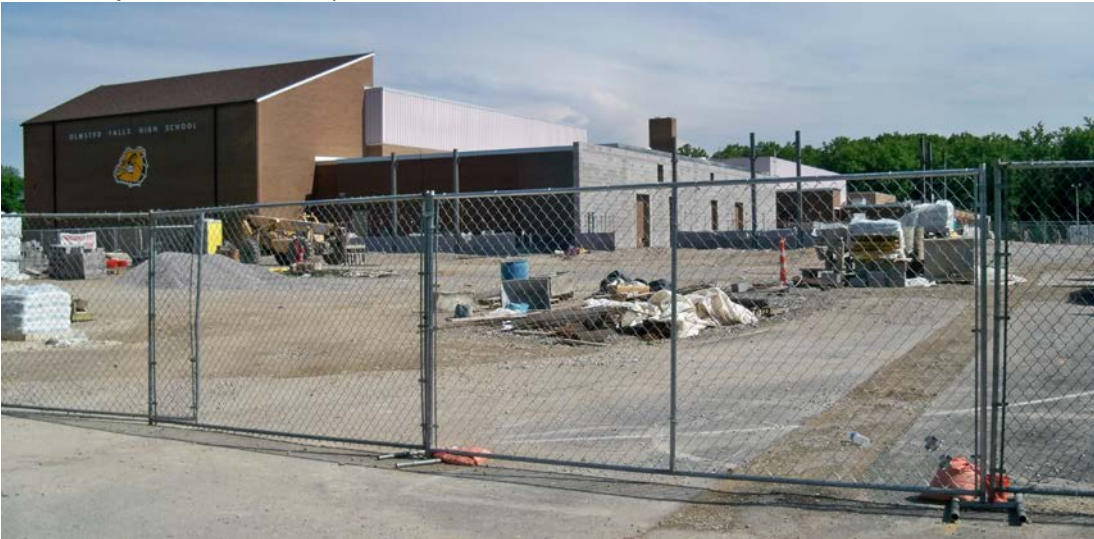
This is another view of construction at Olmsted Falls High School from late May.
